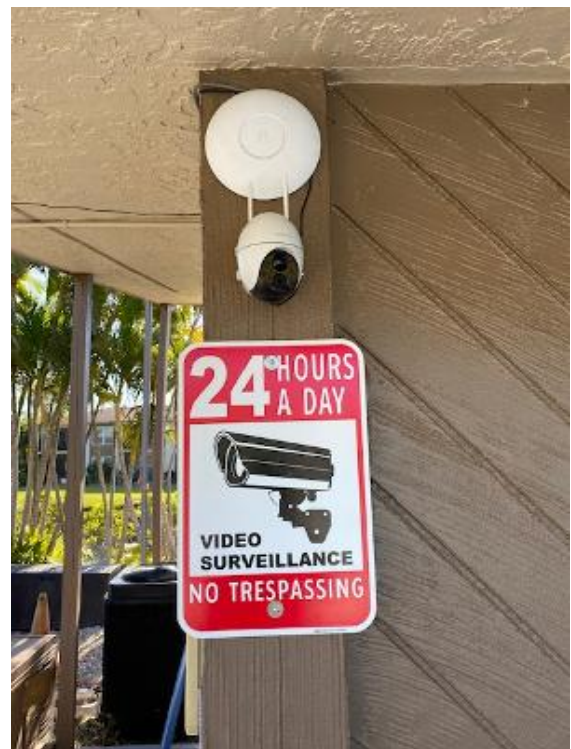
Mounted on the office exterior wall
